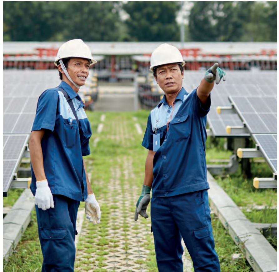
Above: Employees at PMI’s Indonesian affiliate, Sampoerna, solar panel farm in Karawang
